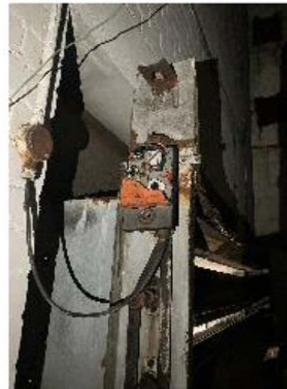
Image 1: Derelict variable intake Louvres
