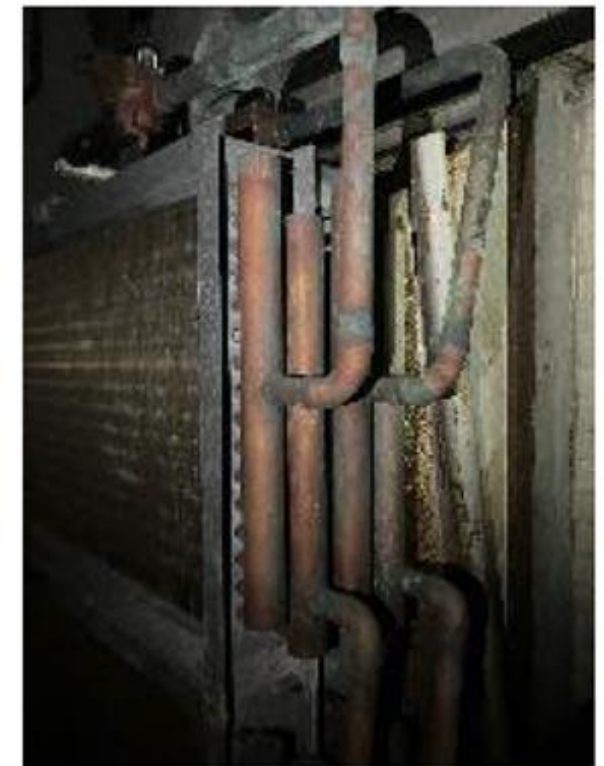
Image 2: Failed Heat-Recovery Coil
